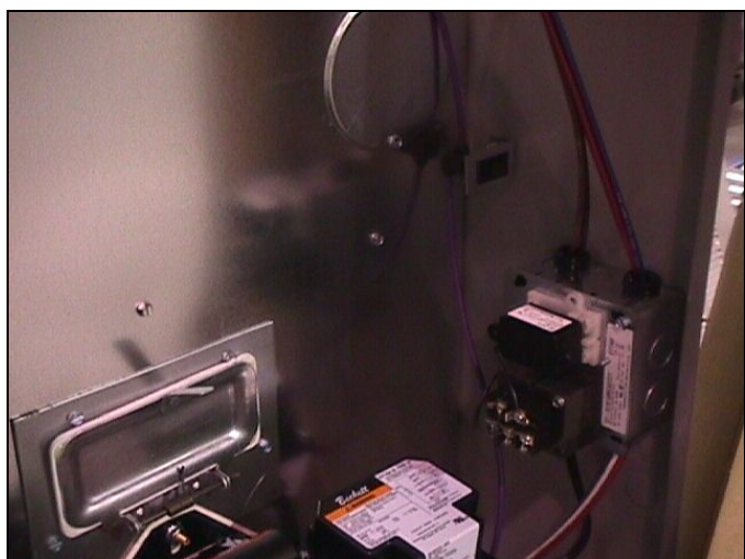
Figure 3: Fan Center and Low Speed Switch
